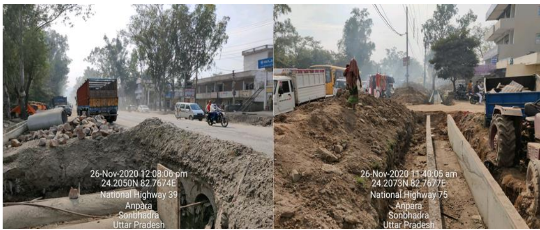
Figure 26: Construction material and debris near construction sites
